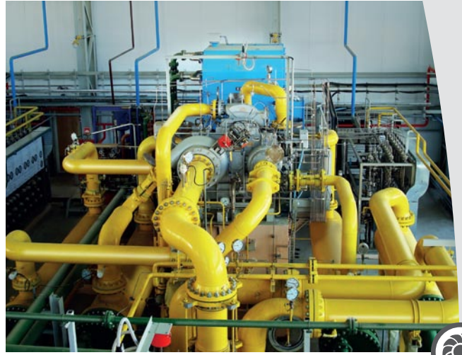
Five-stage centrifugal compressor package
