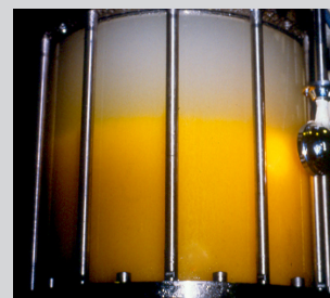
The wash column (ice separator) of a commercial Freeze Concentration plant for orange juice illustrating the sharp separation between washed ice (top) and ice with concentrate (bottom).
