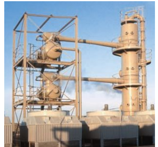
Fig. 9: 3-stage steam jet cooling plant of bridge design, cooling 194 m 3 /hr of water from 28 to 15 °C. Chilling capacity: 2 900 kW
