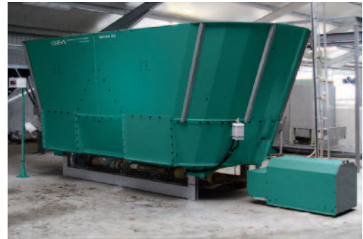
MVM mixer – the heart of the feed supply system
