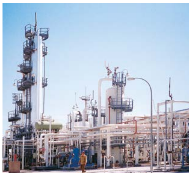
LPG recovery from natural gas by turbo expander cryogenic process. 3,000,000 Nm 3 /day natural gas processing plant.
