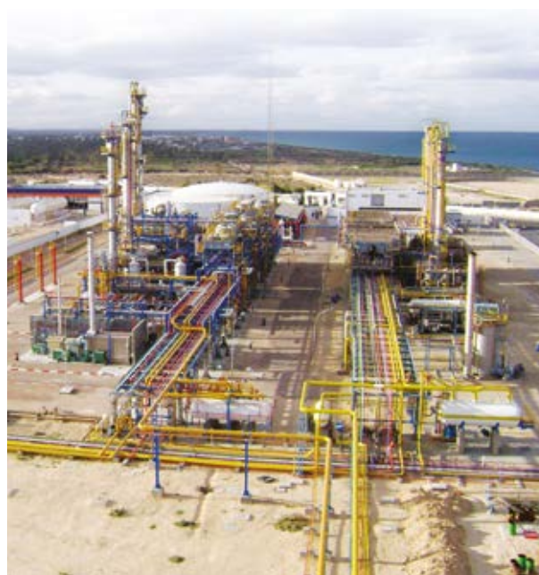
Gas Treatment and LPG Production Plant. 1,250,000 Nm 3 /day natural gas processing and pure Propane, Butane, Gasoline production plant.
