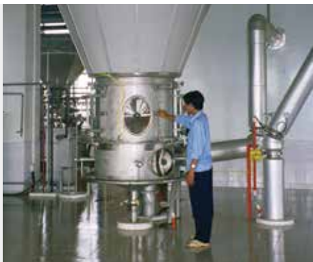
GEA Niro Spray dryer - bottom view
