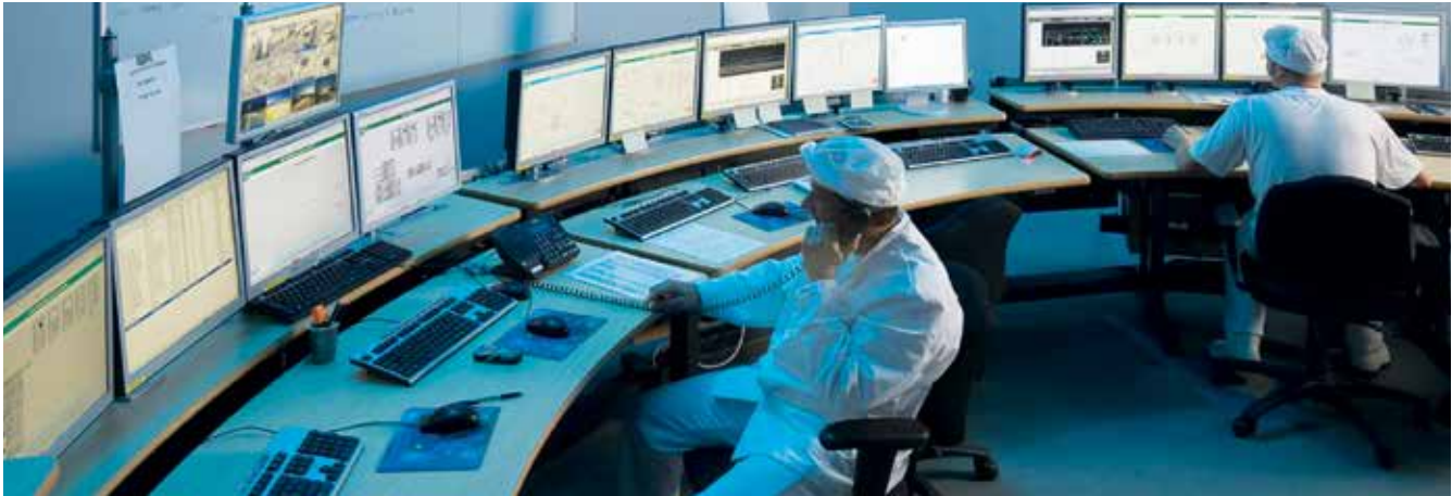
Process control room
