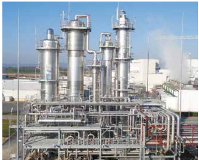
Distillation plant with mechanical vapor recompression for the recovery of solvents from the production of biopolymers
