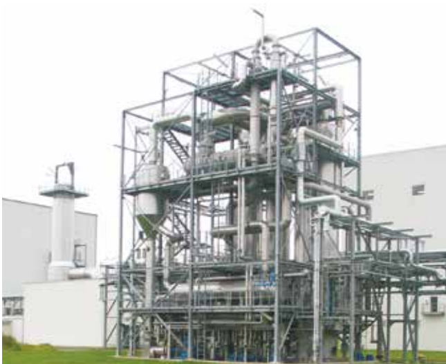
Multi-effect evaporation and solvent rectification system in a pectin extraction plant
