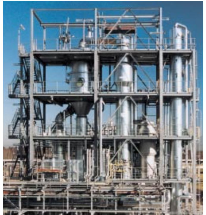
2-effect falling film, forced circulation evaporation plant in counterflow arrangement with downstream system for the purification of vapour condensate by distillation of waste water containing salts and organic compounds. Evaporation rate: 9,000 kg/hr concentrated to 65 % TS
