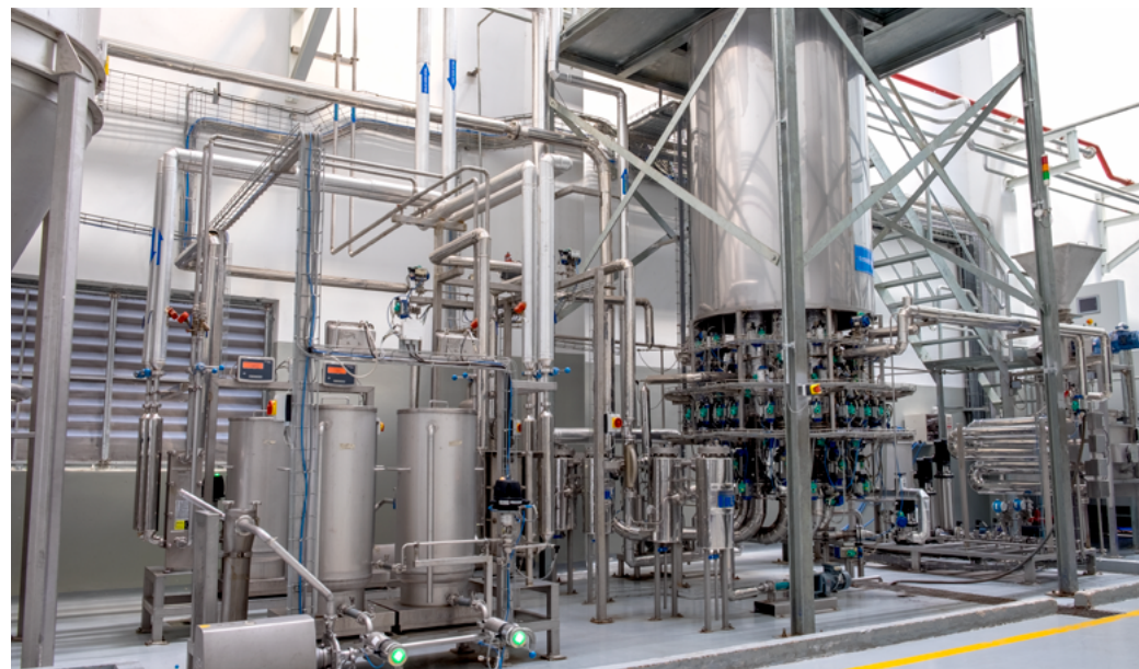
FIC® pilot plant
