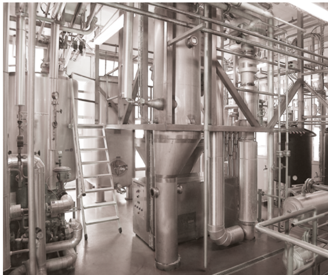
GEA aroma recovery plant
