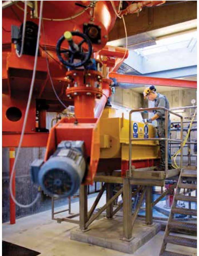
Lime slaking system at a Danish waste incinerator.
