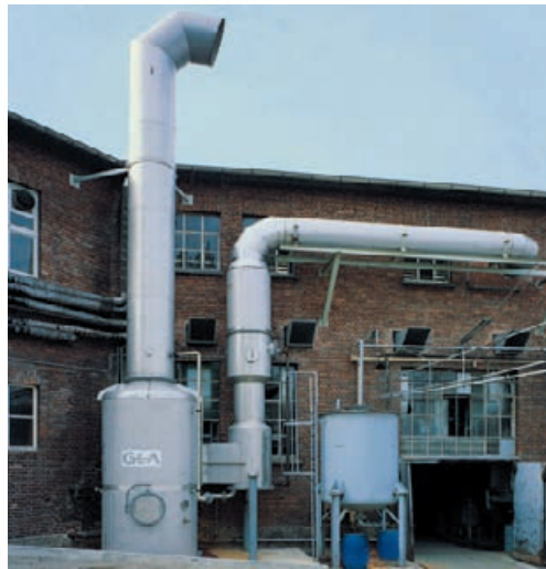
Single effect continuously adjustable Venturi scrubbing plant type U for washing out dusts suction flow: 30,000\ \text{m}^3/\text{h} pressure loss: 20 mbar
