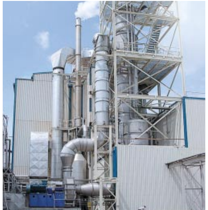
1-effect falling film evaporation plant heated by mechanical vapour recompression for wheat starch effluent. Evaporation rate: 17,000 kg/hr
